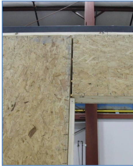
Figure 19. Configuration 5 Failure Mode at Header Panel
